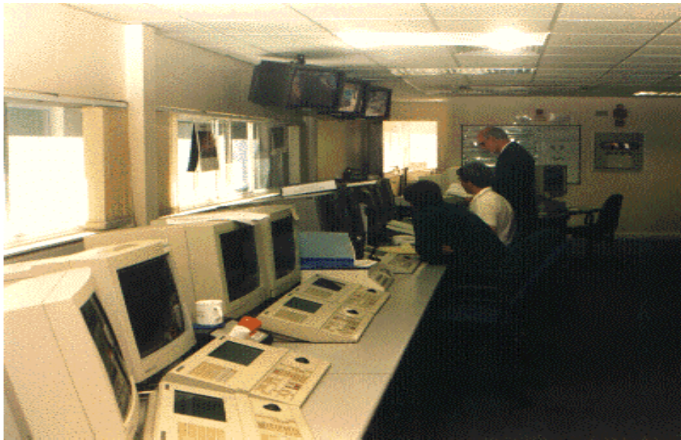
Figure 3: A Typical Control Room
